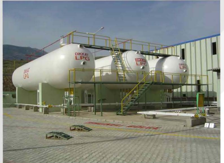
LPG Stoklama Tankı Uygulaması LPG Storage Tanks Application
